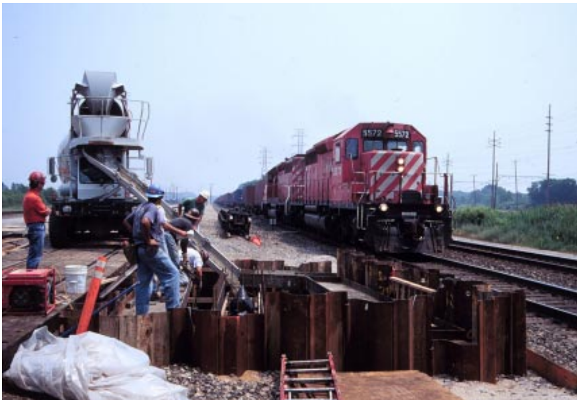
A westbound CP train passes a construction crew at Burns Harbor, IN, on the NS (former CR) Chicago line. CP engine 5572 in the lead. This will be the location of a new overhead bridge for Route 249. Photo by Rick Schroeder, 6-24-99.
